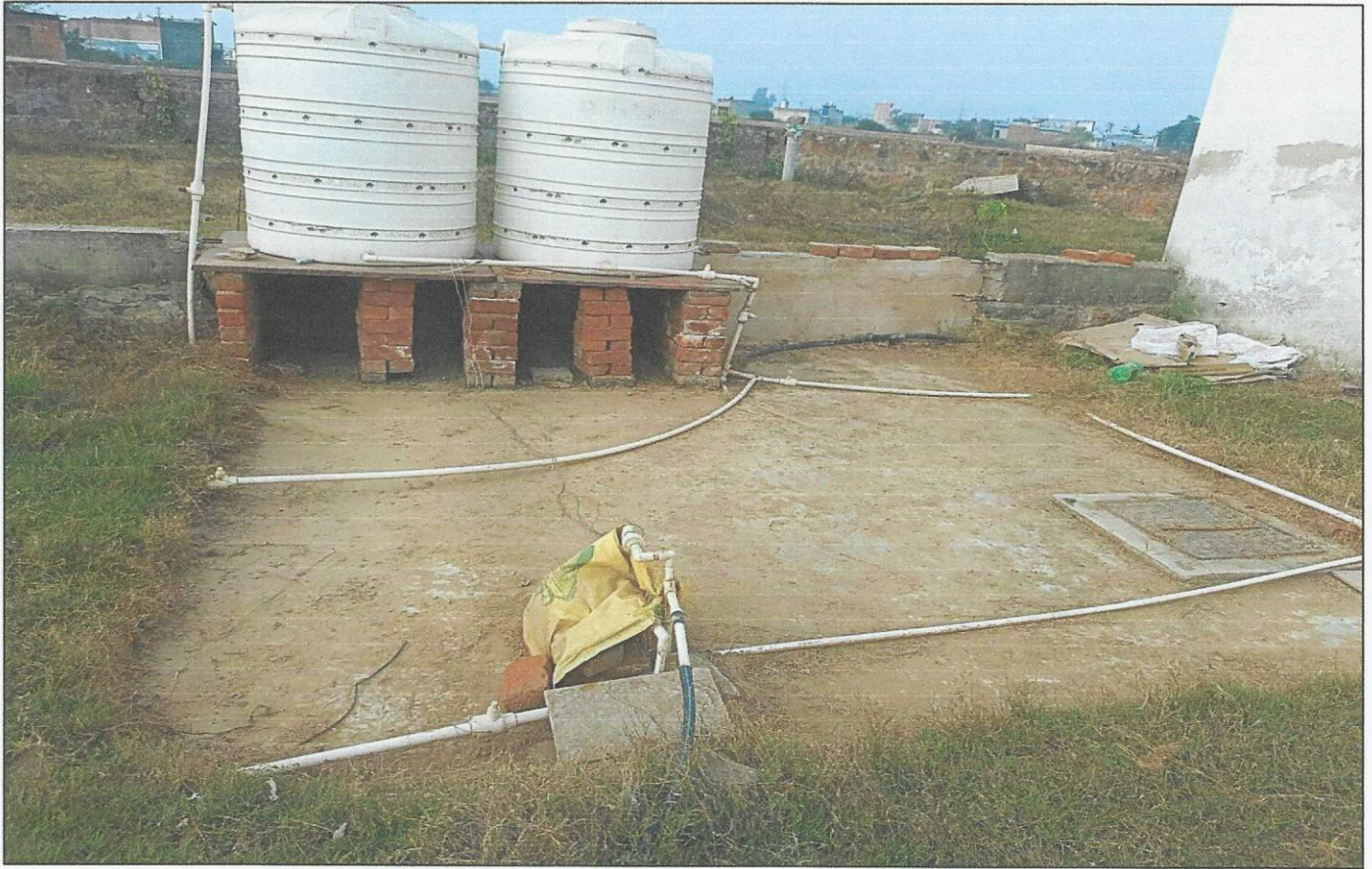
UNDERGROUND WATER TANK
