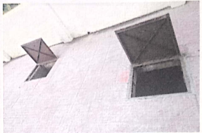
RAIN WATER HARVESTING
